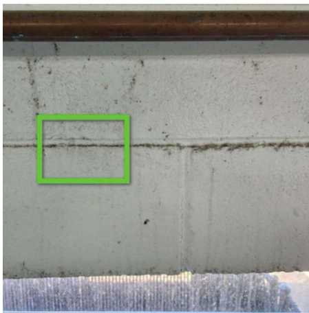
Downstairs kennel middle left side wall
