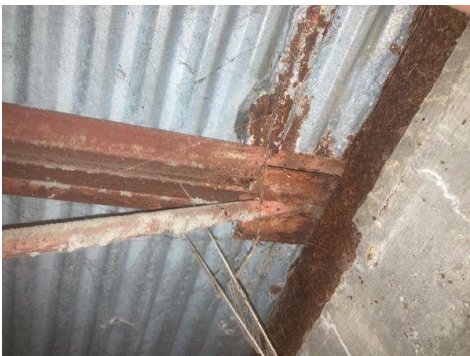
2.1.7 Exterior Distress MODERATE CORROSION ON STEEL JOIST CENTRAL AND NORTH CONCRETE WALLS
