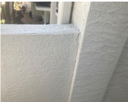
Exterior Distress: Siding separation
