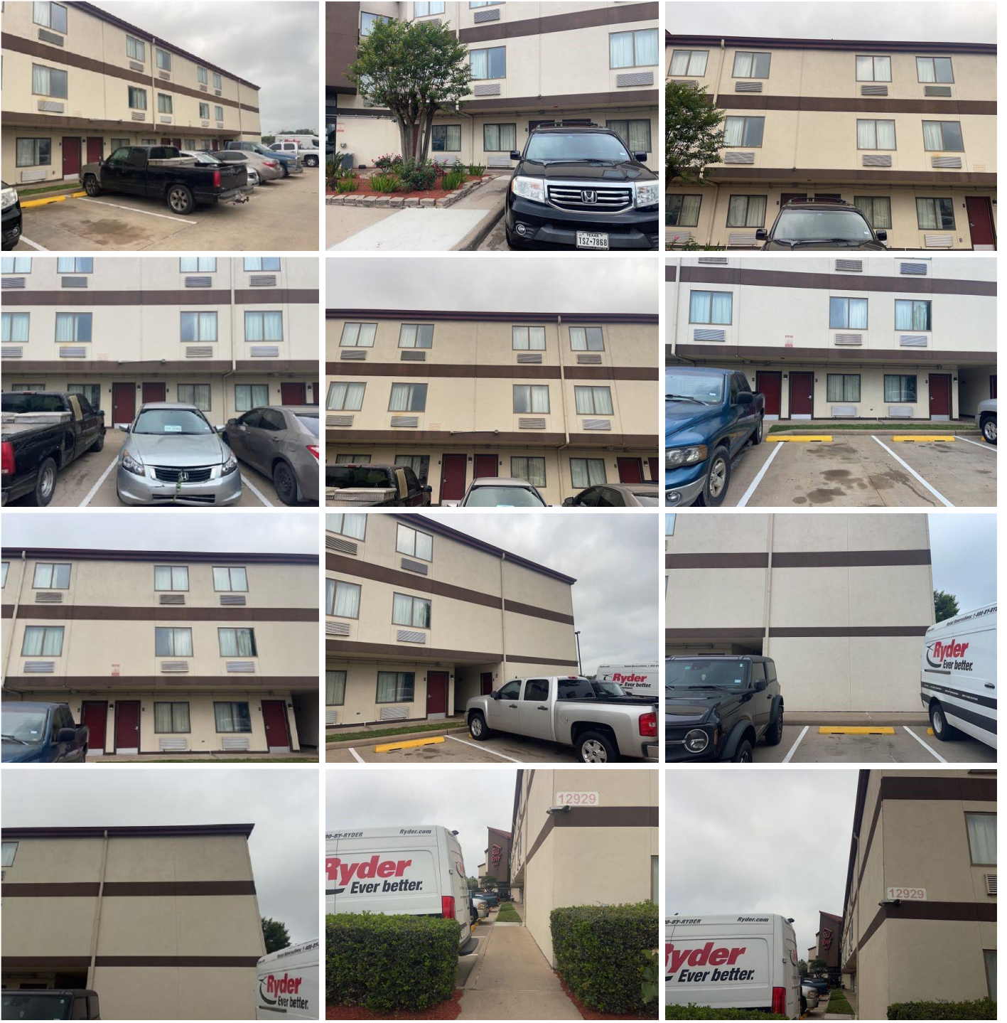
Exterior Distress: Stucco Veneer Cracks
