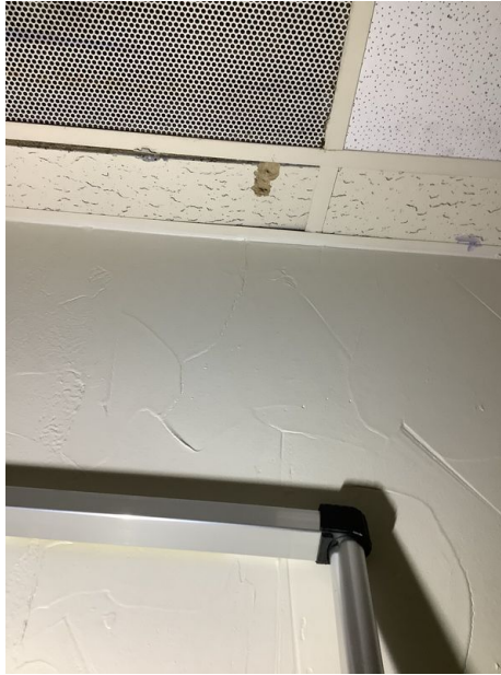
Pin & fissure ceiling tile
