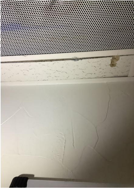
Pin & fissure ceiling tile
