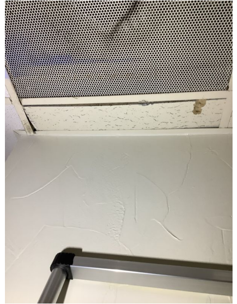
Pin & fissure ceiling tile
