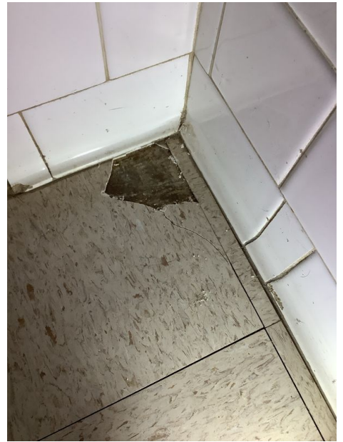
Tan floor tile & mastic
