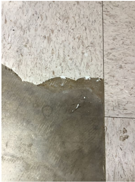
Tan Floor Tile & Mastic
