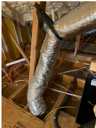
Filter Type: No Filter Filter Location: At Unit(s) in Attic Filter Size: Not Observed
