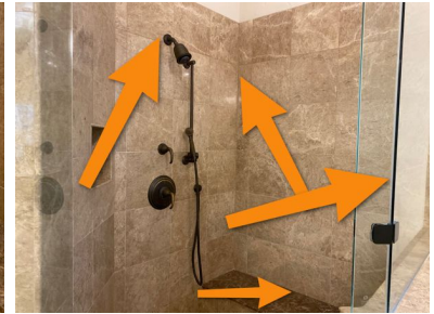
Master/Primary Hers Bathroom
