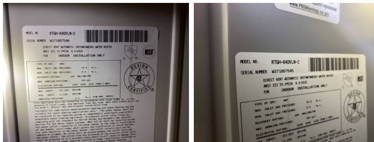
General Mechanical Photos:
