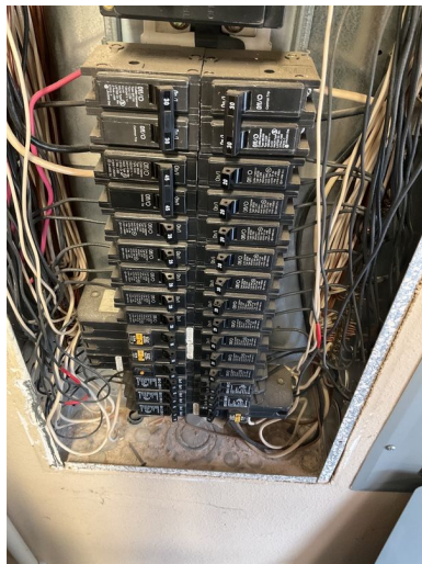
Electrical Service Entrance: Underground Panel Location : Exterior Panel Brand: Cutler - Hammer
