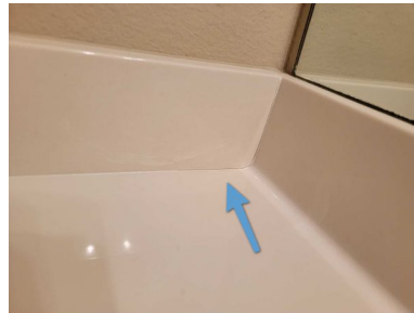
Upstairs Middle Bathroom
